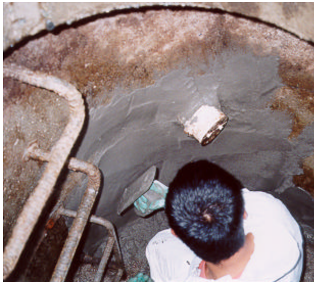
Figure 2. – Trowel application of patching material in manhole on Marine Drive (August 2001). Photo by Jon Walter
