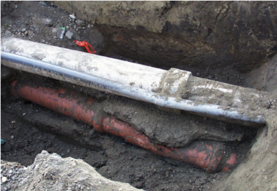
Figure 3. On Marine Drive, broken 12" diameter clay sewer pipe below water pipe and electrical conduit. (September 2001) Photo by Jon Walter
